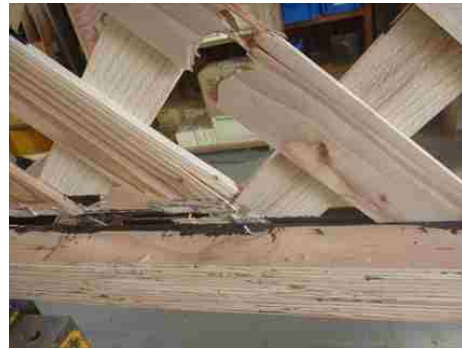
Fig. 3-9 Typical failure in 1P-28-41
